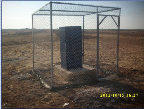
Ground Water Station Mahasi, AL-Ramtha TeWaRON 3
