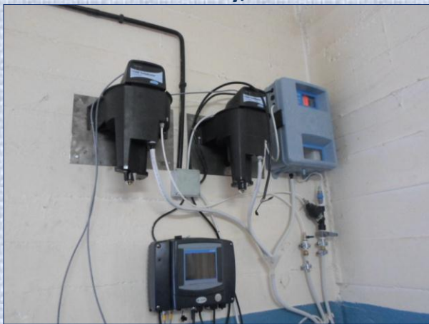
Turbidity & Chlorine In Water Spring Measuring Station, Ajloun.
