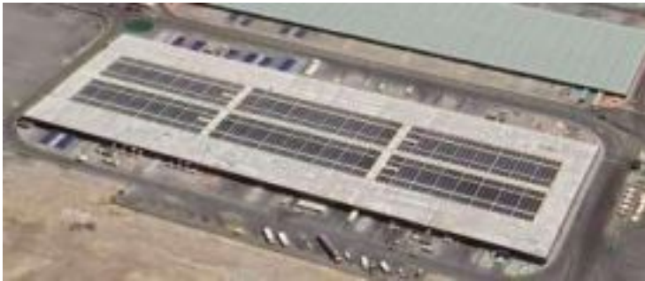
1.75 MW PV PLANT – AMAZON WAREHOUSE, JEDDAH – KSA
