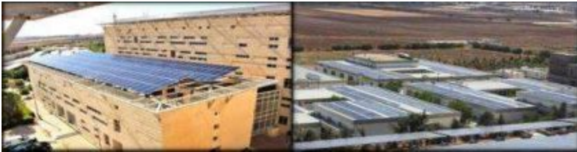
Rooftop Solar Systems
