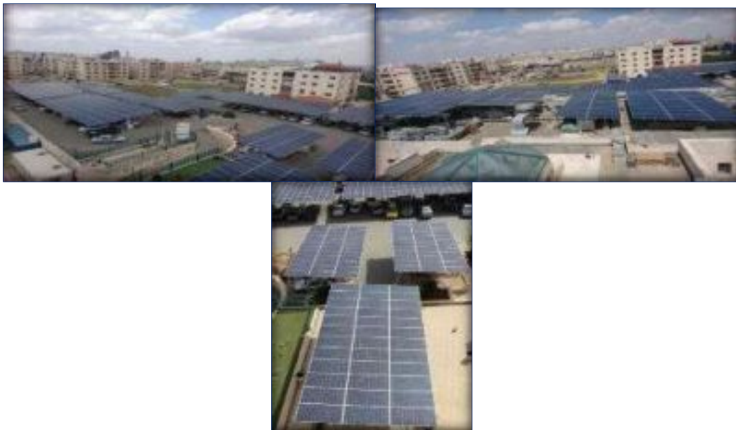
0.804 MW PV PLANT – IRBID SPECIALITY HOSPITAL
