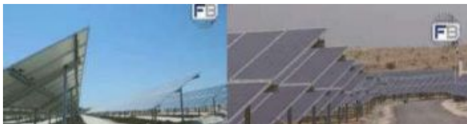
Ground-Mounted Solar Power Plants
