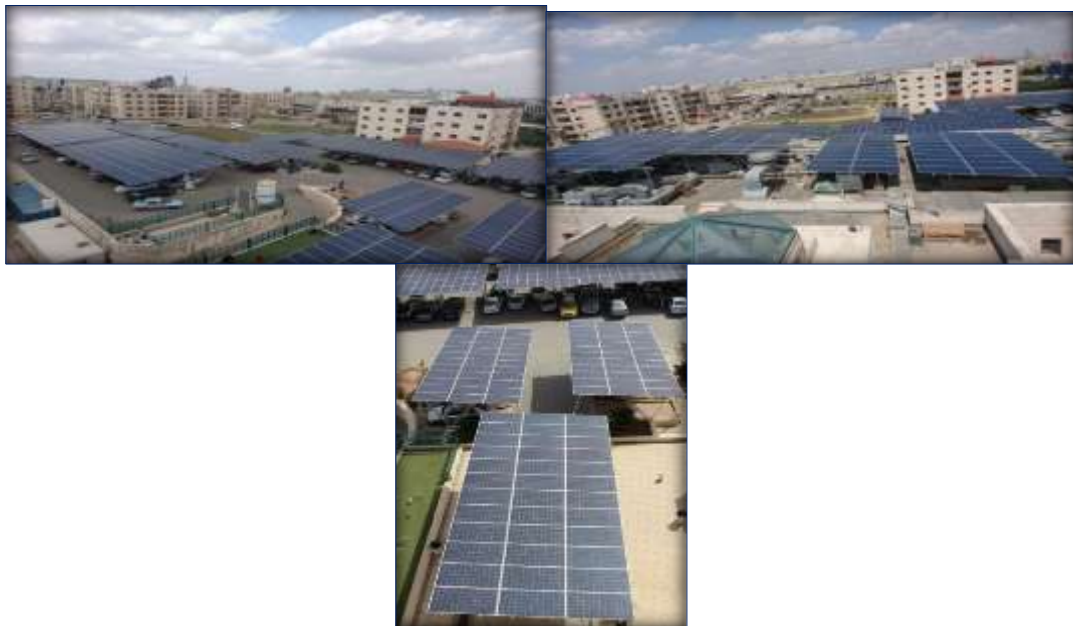
0.804 MW PV PLANT – IRBID SPECIALITY HOSPITAL
