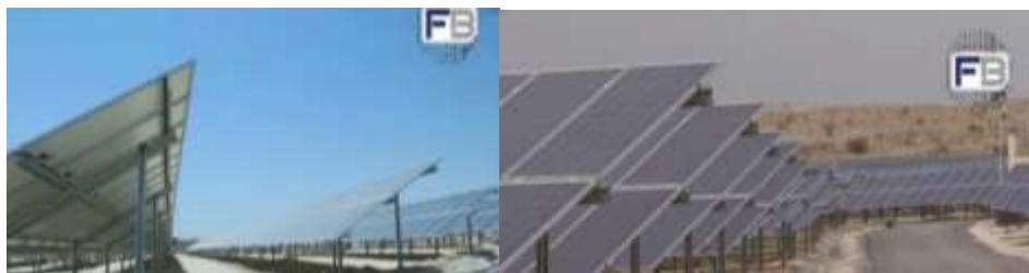
Ground-Mounted Solar Power Plants
