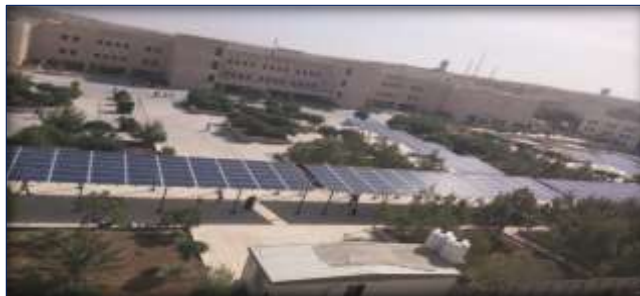
5 MW PV PLANT – HASHEMITE UNIVERSITY
