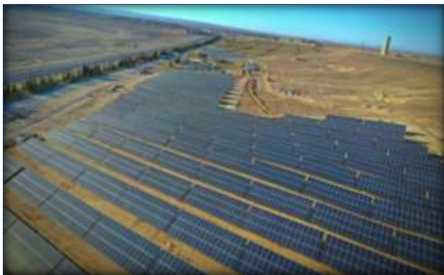
3 MW PV PLANT – AL HUSSEIN BIN TALAL UNIVERSITY
