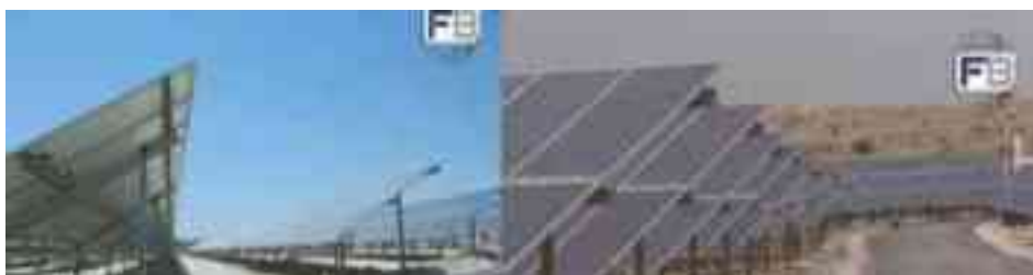
Ground-Mounted Solar Power Plants
