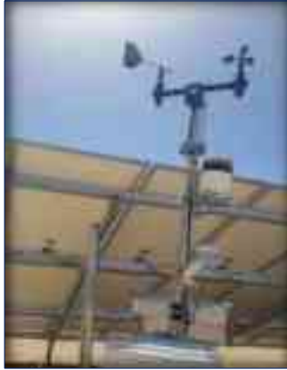
Automatic Weather Station Al Hussein Bin Talal University, Ma'an Integrated with 3 MW Solar Energy Plant
