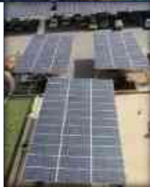
0.804 MW PV PLANT – IRBID SPECIALITY HOSPITAL
