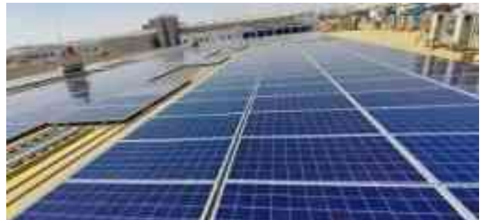
1.4 MW PV PLANT – IKK GLASS FACTORY, JEDDAH – KSA
