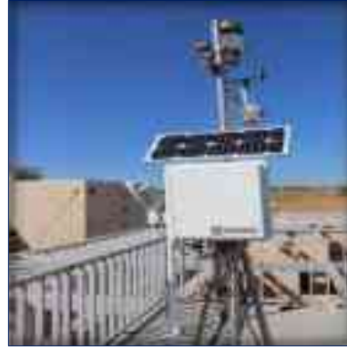
Automatic Weather Station German Jordanian University, Madaba Integrated with 2.11 MW Solar Energy Plant
